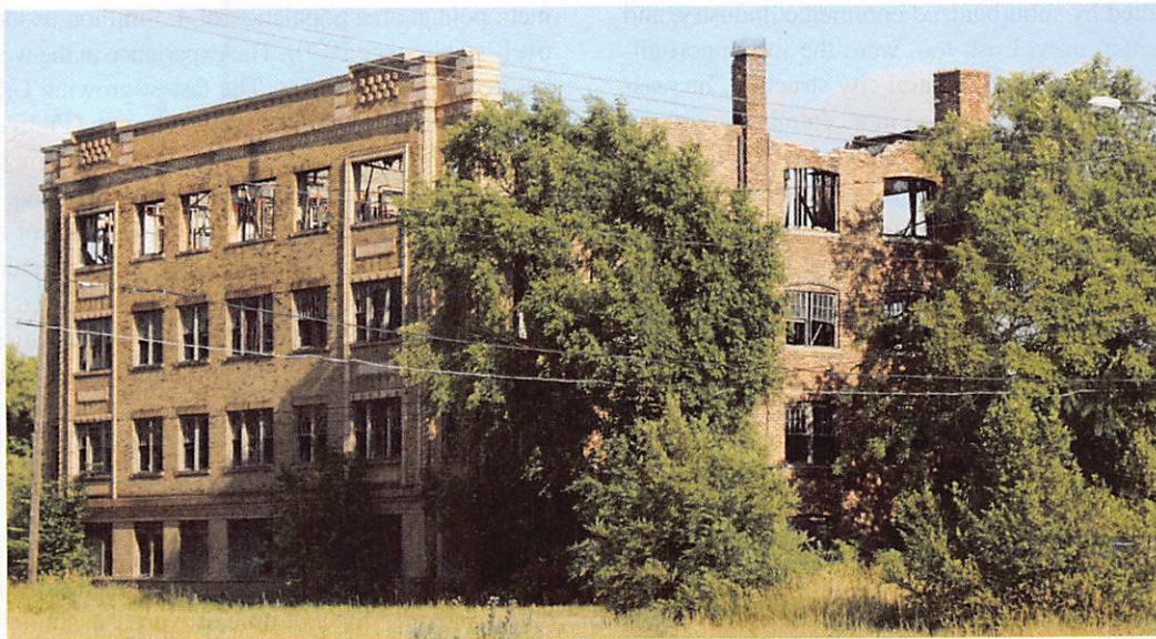
Figure 11.32 Abandoned housing is common in Gary, Indiana as a result of white flight and deindustrialization. Some areas of cities have witnessed significant disinvestment and population decline. Properties in such neighborhoods have such weak resale and redevelopment potential that owners abandon them. Buildings left to decay become a source of danger and blight for those that remain. Since its peak in 1960, Gary has lost more than half its population.
